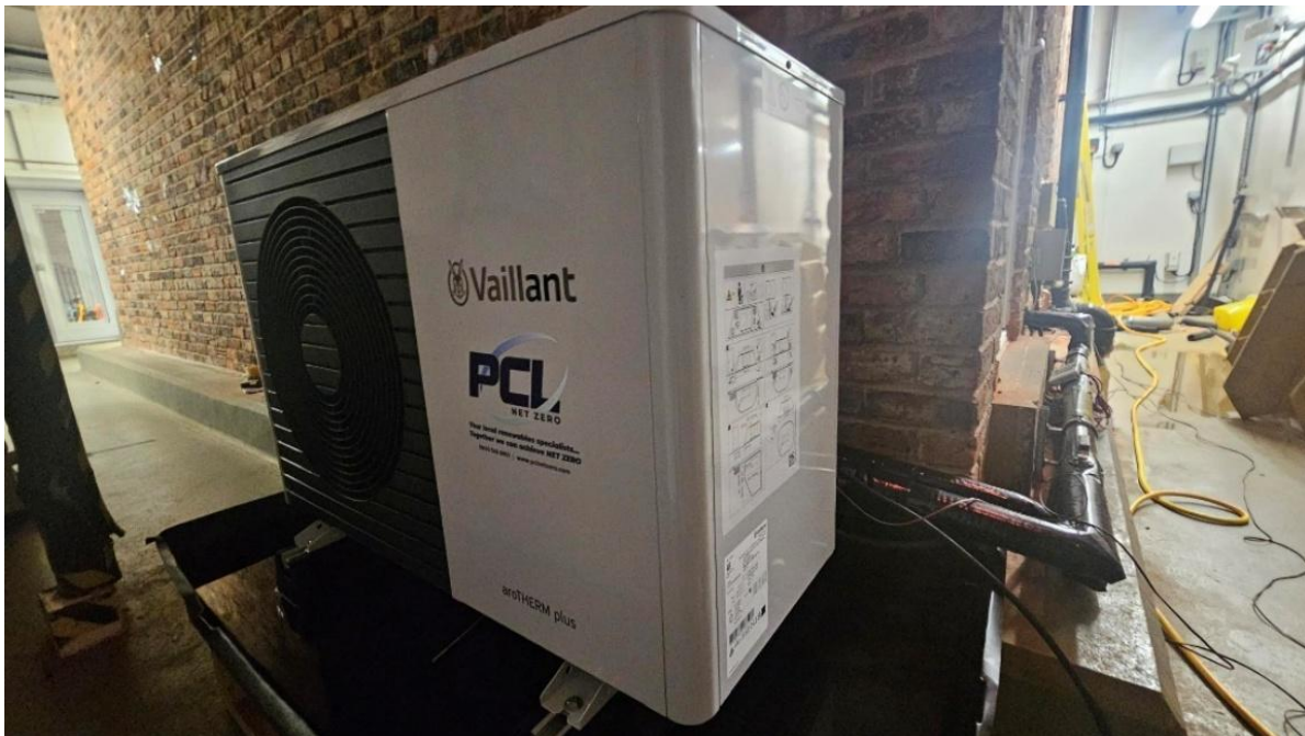
Figure 1: Vaillant aroTHERM plus ASHP installed for the test.
