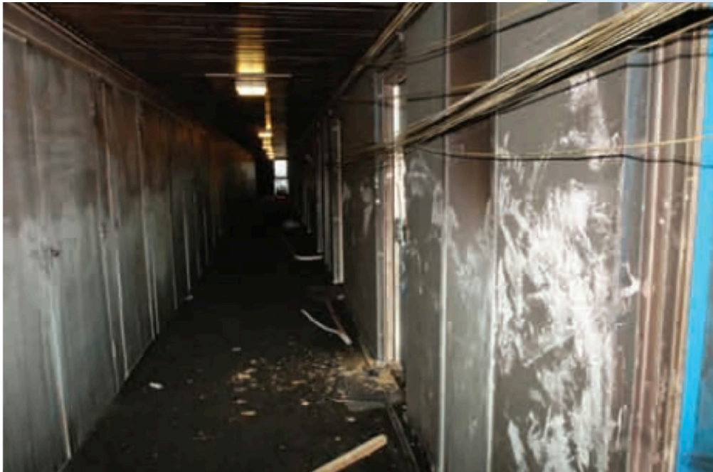
Post-incident photograph showing conditions on the eleventh floor after the escape door from Flat 27 was left open, note the displaced cables.
