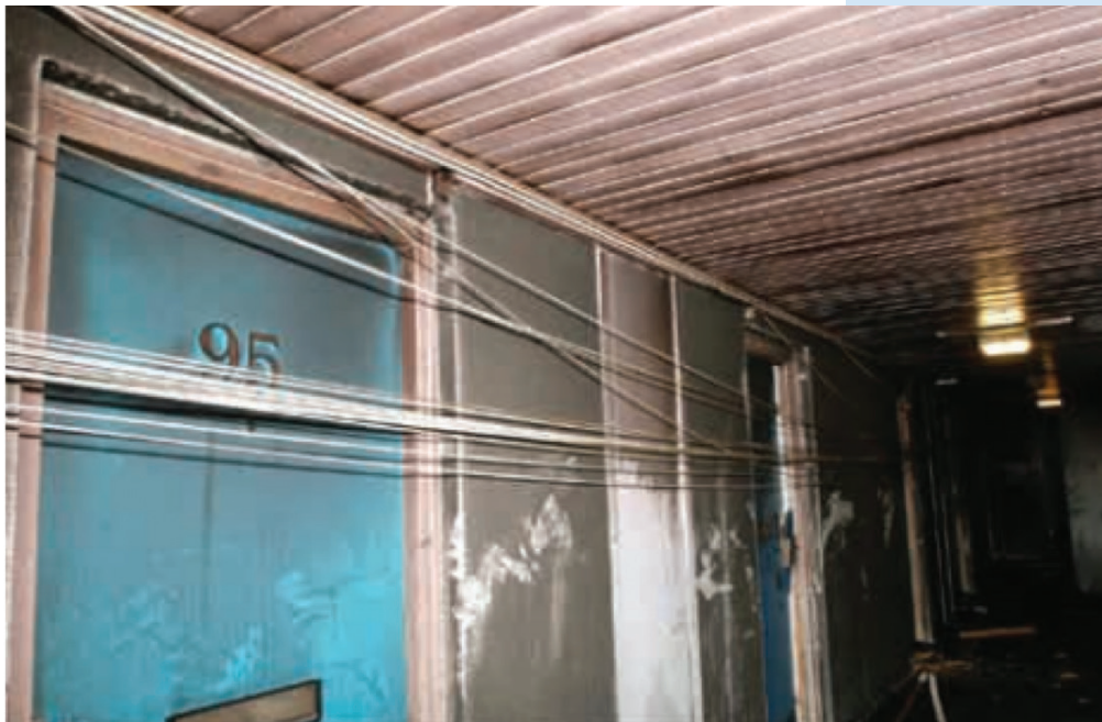
Post-incident photograph of the eleventh floor landing showing displaced cables.
